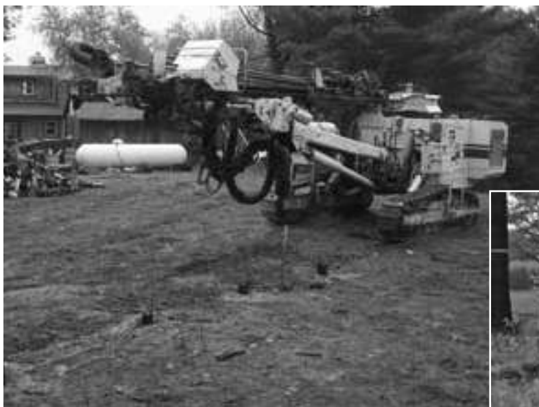
Left photo: Holes have been drilled 20 feet deep for the dynamite charges. photo by Rob Robertson
